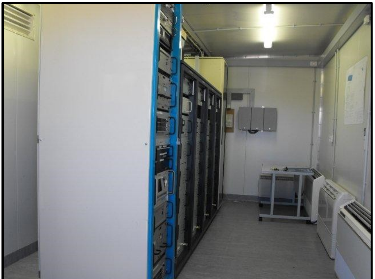
HF transmitting room
