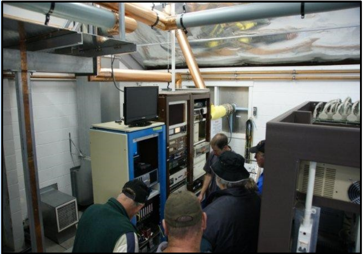
Transmitting Room Rangitaiki Marine HF transmitting Station
