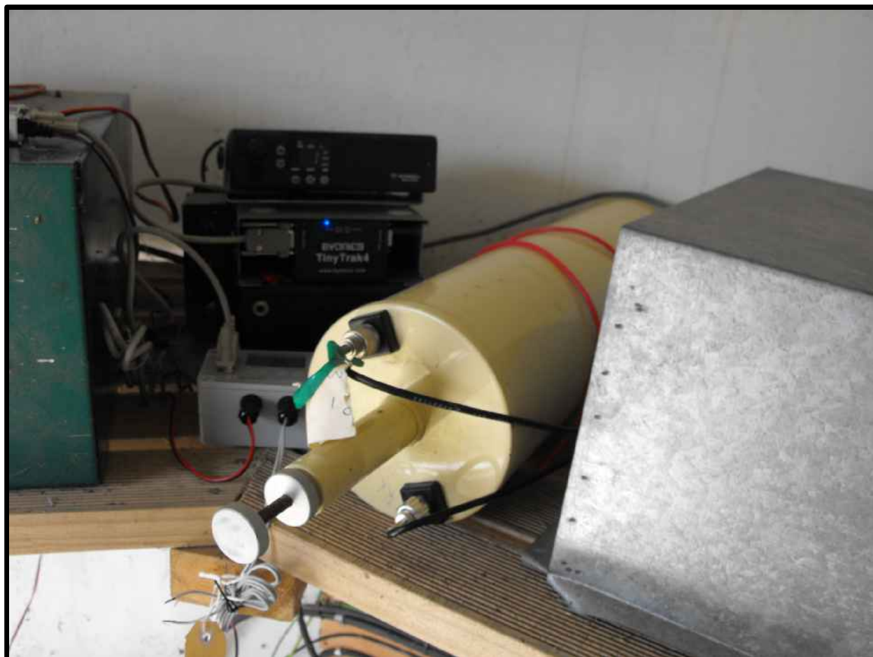
APRS equipment (black) nestled amongst the commercial radio gear at Mt Misery, Northern HB
