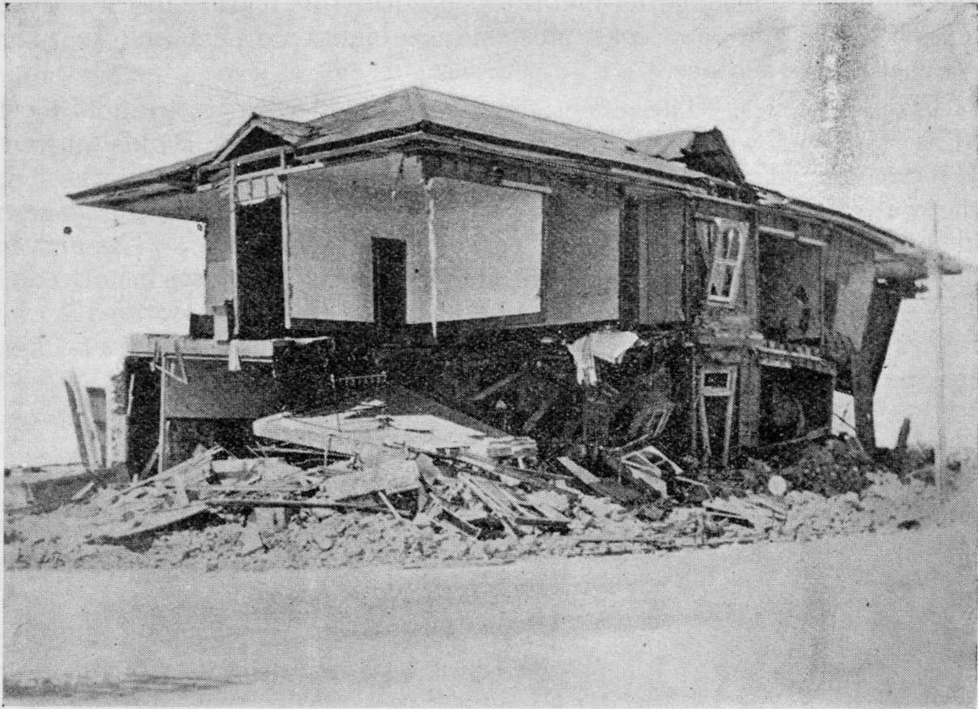
FIG. 2.—Brick building damaged through use of poor-quality mortar, and inadequate tying of interior partitions.
