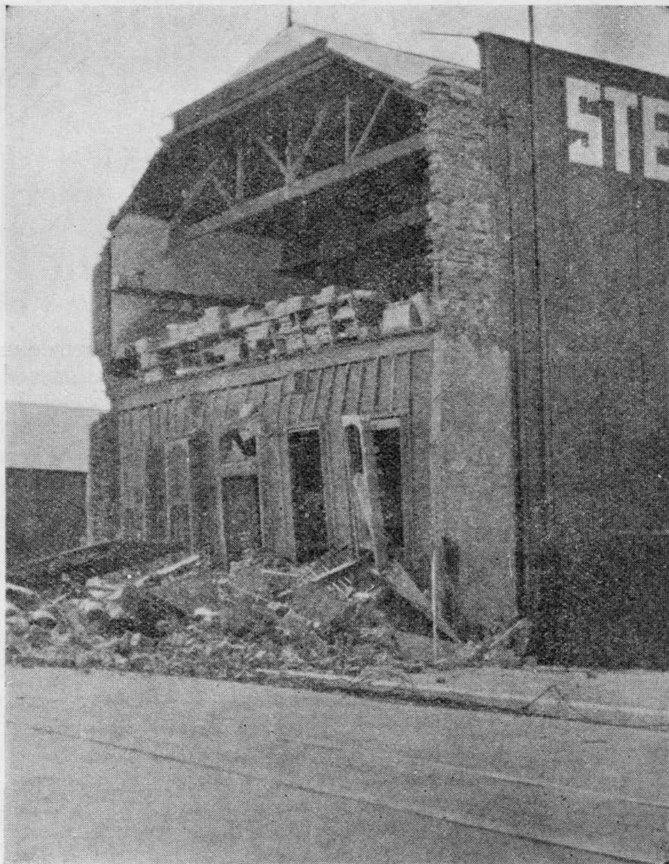
FIG. 3.—Collapse of brick façade inadequately tied to building.
