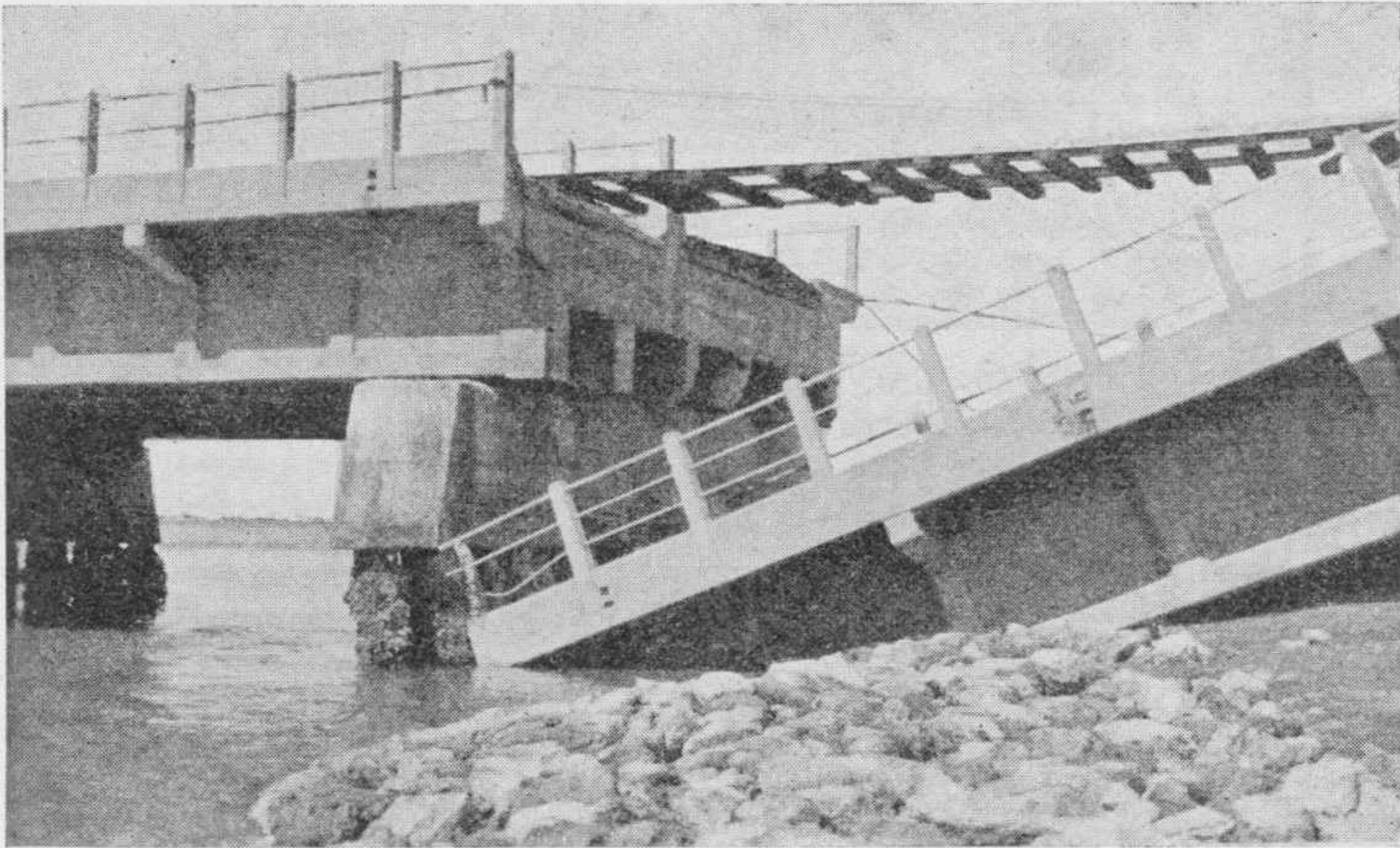
PLATE IV.—(c) West Shore bridge, Napier. The mud-bank to the right of the channel slumped and forced a group of piles from under the end of the span.
