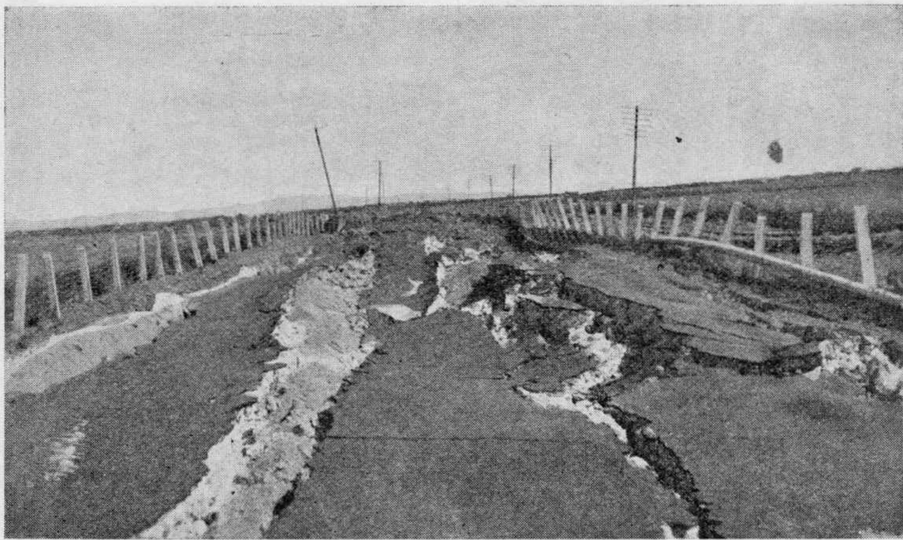
PLATE IV.—(b) West Shore Causeway, Napier. The embankment spread laterally.
