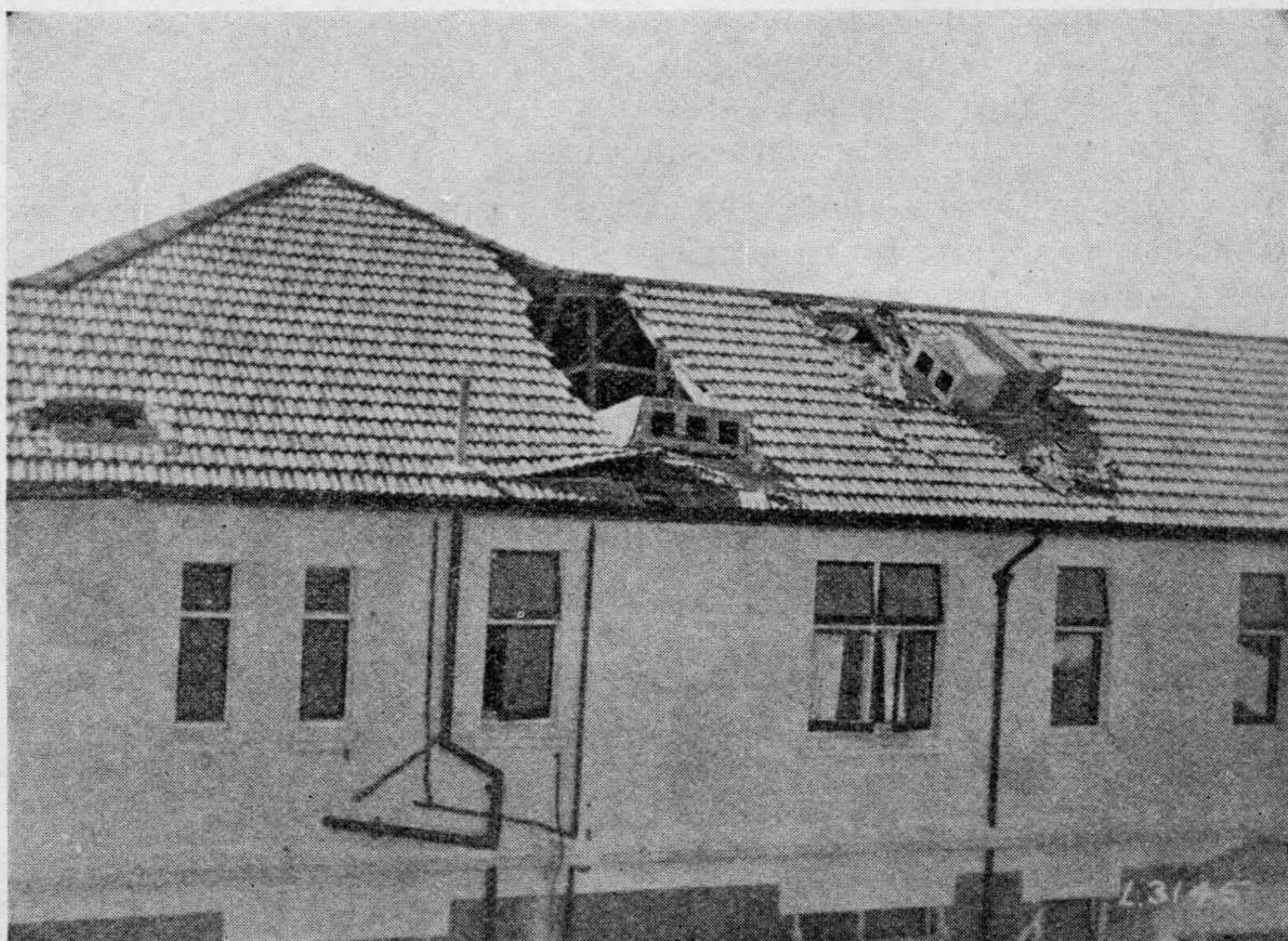
FIG. 1.—Damage caused by collapse of massive chimneys.
