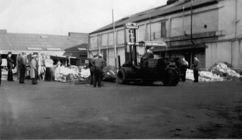
Tuck Bros (Napier) Ltd. - Bullmoose Forklift (9ton lift) Demolition of Hawke's Bay Motor Company building Dicken Street Napier. : Photo 1956.
