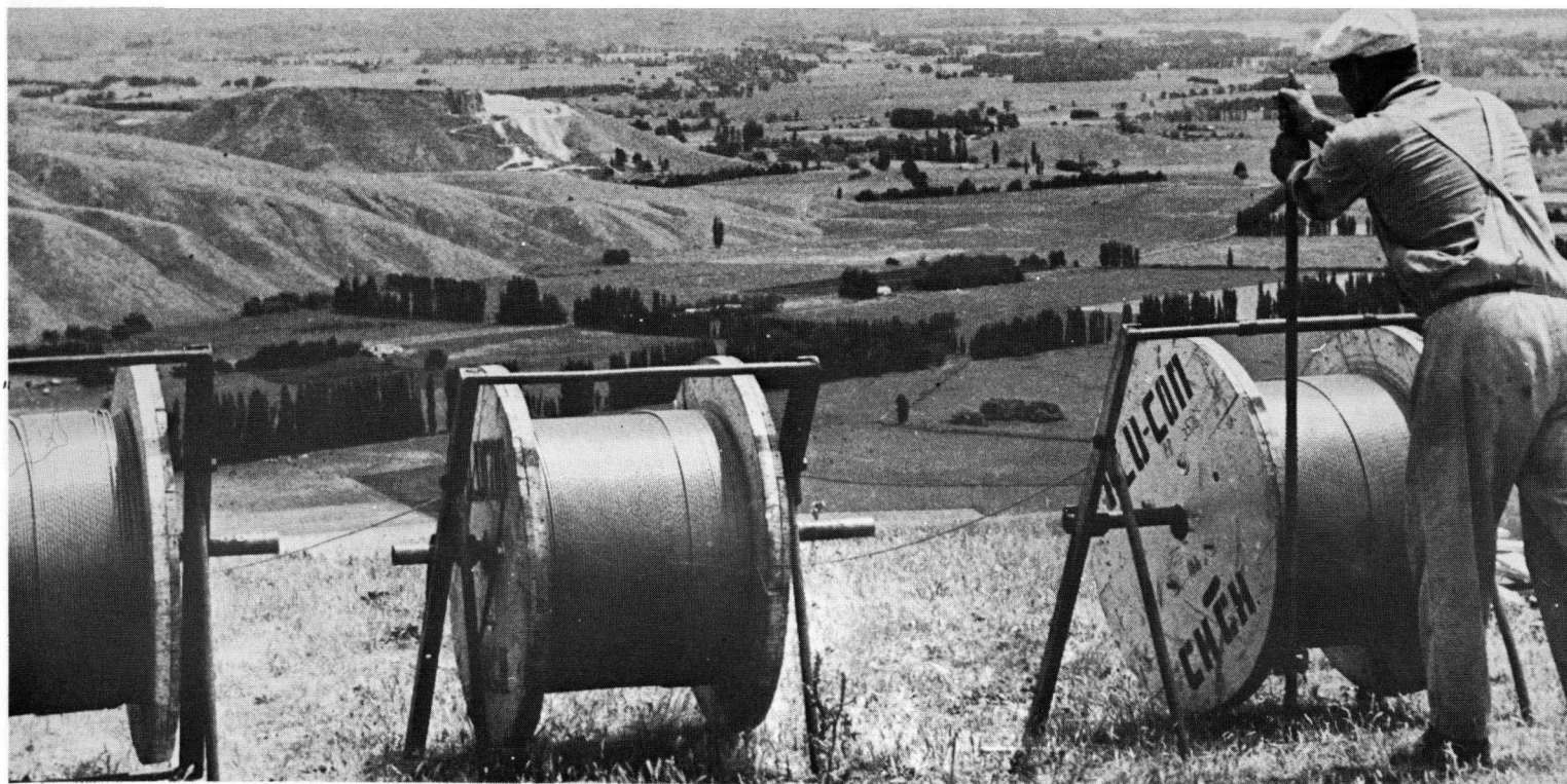
The introduction of television to Hawke's Bay entailed the supply of electric power to the Mount Erin translator. Here lineman Mr D. Reid is steadying a cable drum as lines are run down the steep hillside — M. Leete.
