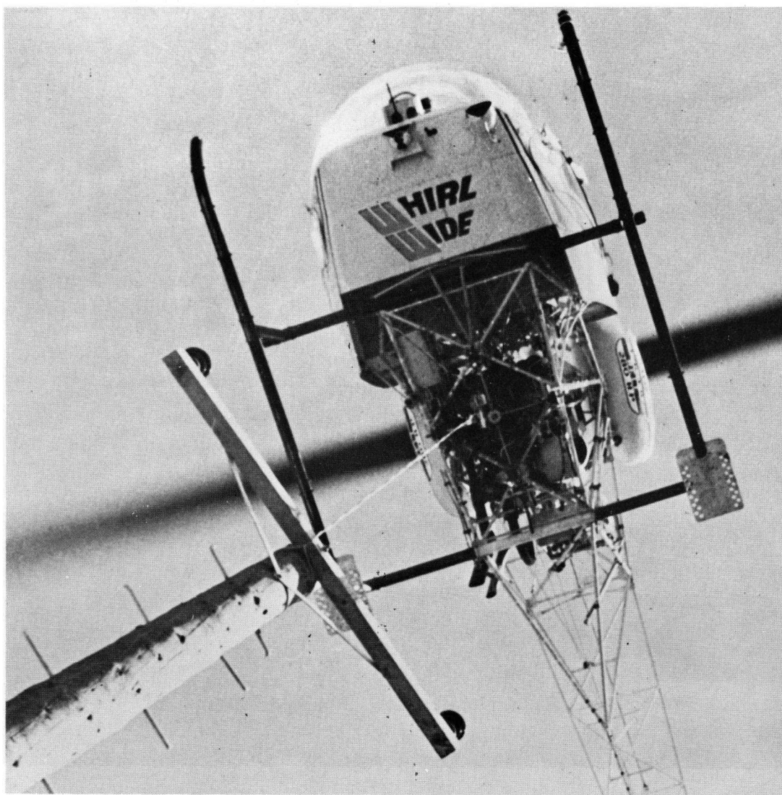
Erecting poles and cabling in rough country can be back-breaking, tedious and expensive work. In 1972 at Taraponui on the East Coast the board used this helicopter to transport poles and lower them directly into pre-dug holes on the hilltops.
