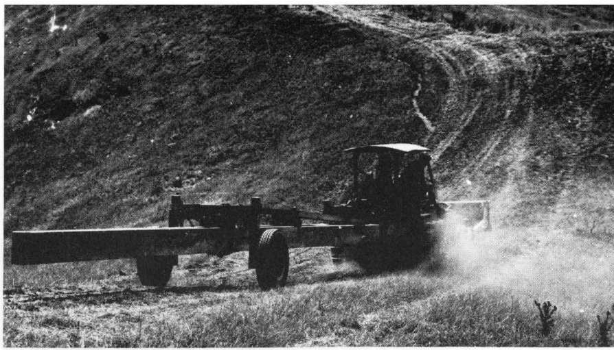
Caterpillar tractor makes light work of hauling heavy concrete pole up steep grades.
