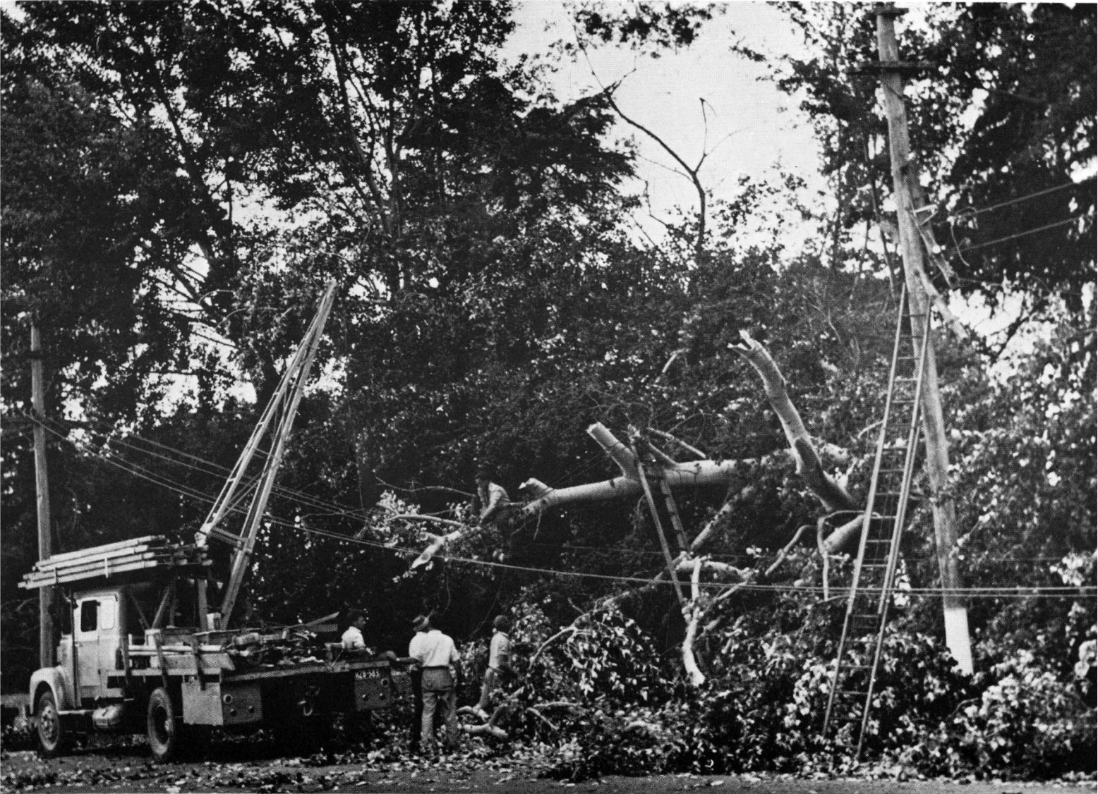
Falling trees play havoc with Board's reticulation services. This mess kept a line gang busy for a day.
