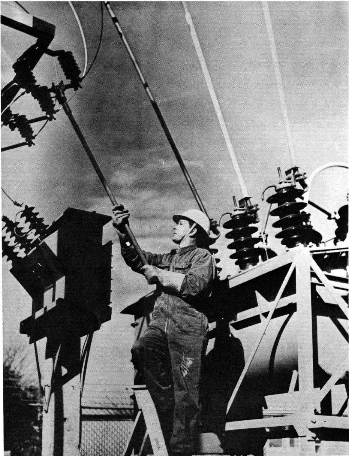
Mr M. Bell in hard hat pulls high voltage fuses. — M. Leete.
