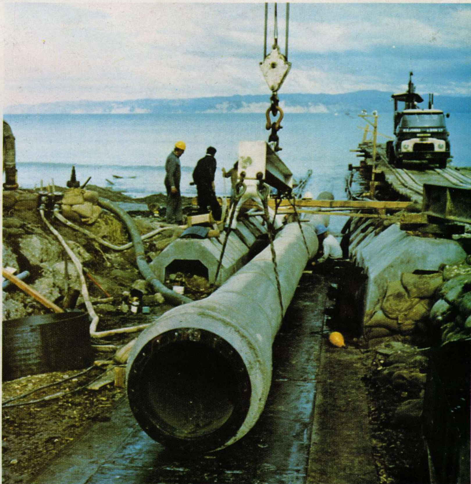
The laying of the sea outlet pipe for the Gisborne Refrigerating Company's new effluent disposal system (story page 3).
