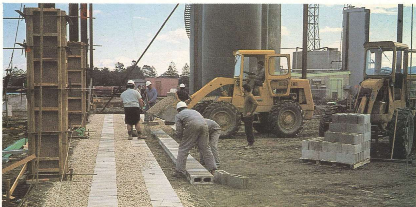
Laying the underfloor ventilation which will prevent frost heave under the building.
