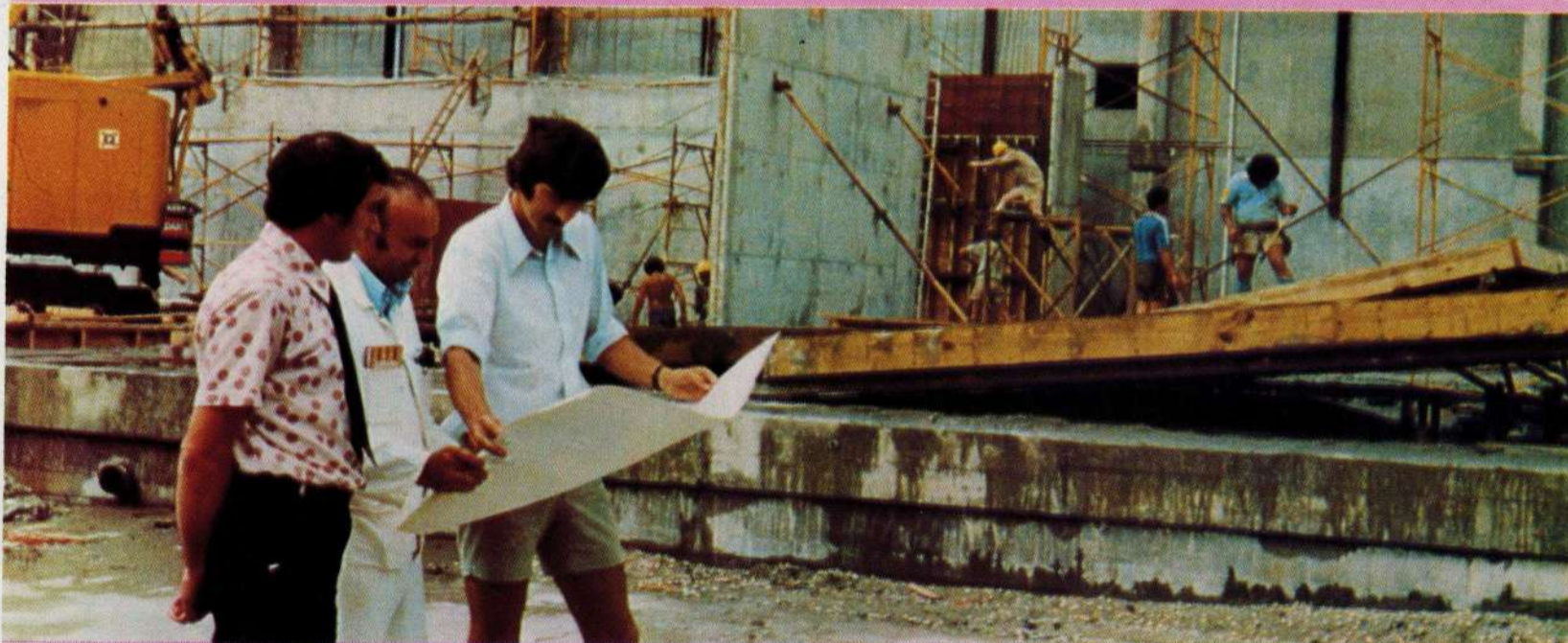
Site Engineer Nigel Whiteman following the early progress at the new freezer area with the Kaiti chief engineer Clive Jepsen and Ron Clayton, foreman at the carpenter's shop.
