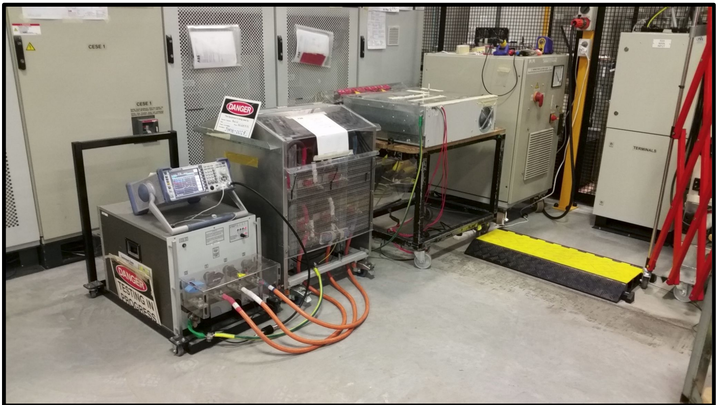
ABB test set up for conducted RF emissions test
