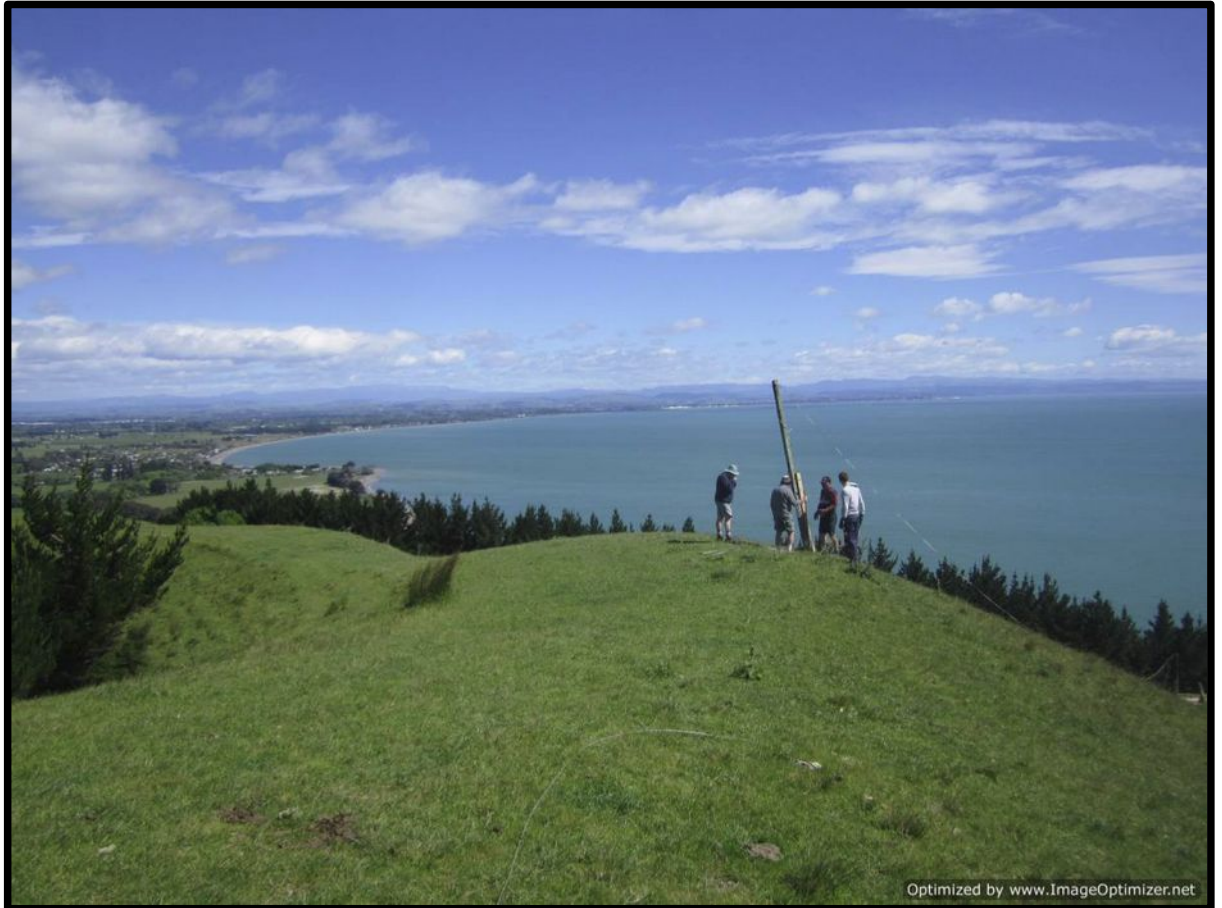
Some of the Team erecting a new HF aerial for the Clifton accessor
