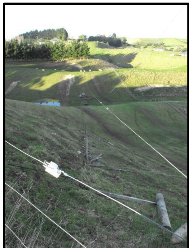
showing the long leg of the OCFD across the valley to where the sheep are
