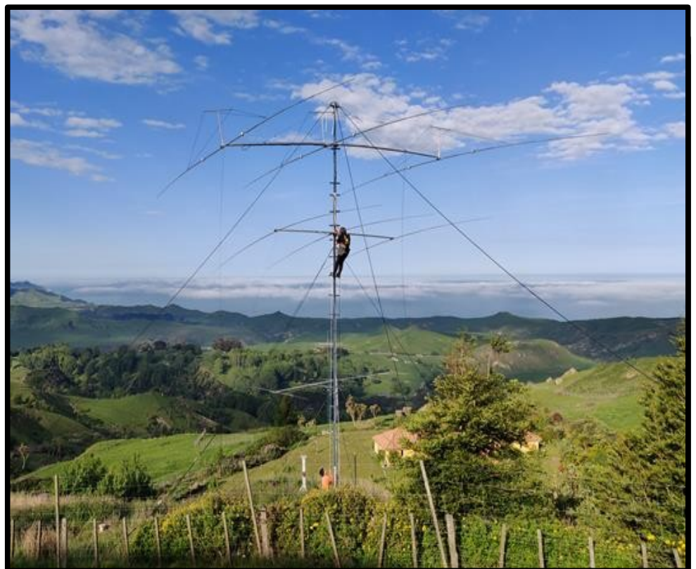
Jaidyn - ZL4WW - in action on the tower, Alec - ZL1HAZ - seen at the base as ground crew
