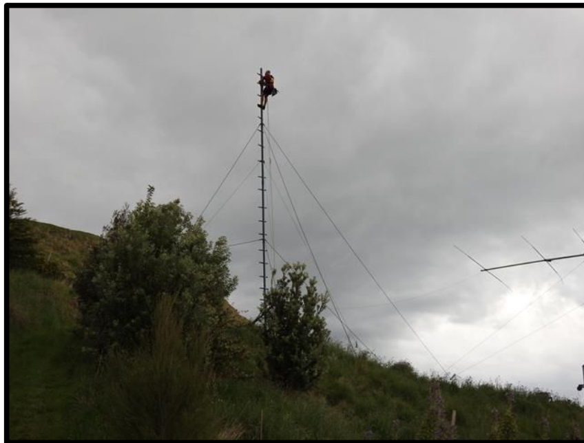
Figure 5: Oct-2019, Marek-OK1MV on the tower installing the gin pole for the next segment
