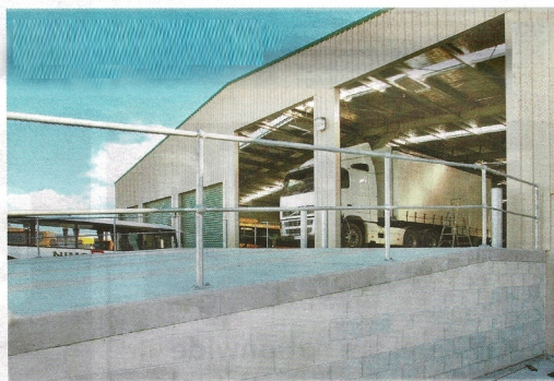
Ramp up to the workshop where mechanics service the buses and commercial clients.
