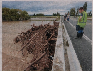
Slash on the Tutaekuri River bridge on the Hawke's Bay expressway.
