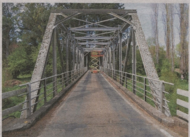
Rissington Bridge on Puketitiri Rd in Hawke's Bay, which had only recently undergone strengthening, was this week completely destroyed in flooding from Cyclone Gabrielle.
