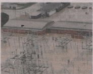
Detail from an aerial shot of the flooded Redcliffe substation.
