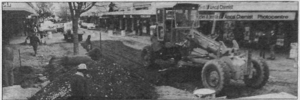
Graders and excavators tested the patience of shopkeepers and motorists alike while the central-city redevelopment took place. Underground services should not need attention for the next 20 years.
