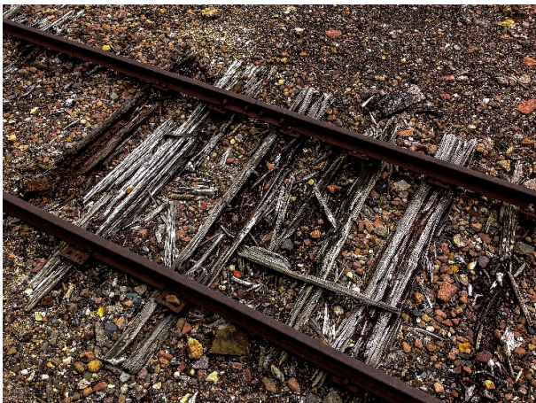
Caption: The corroding railway lines at Buchenwald Camp, 2014. (Photograph courtesy Glenys Scott)
