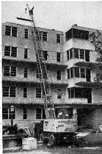
A Coles with 60' jib and 12' fly jib handles building components for a block of flats in Canada . . .
