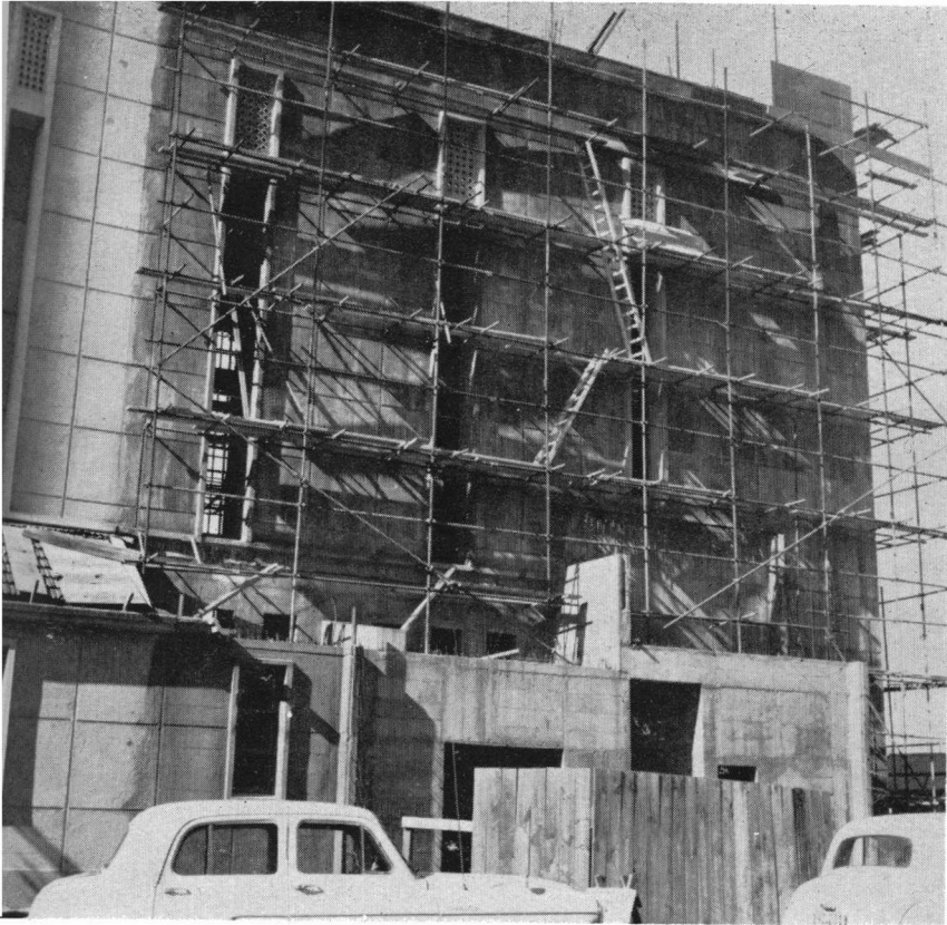
The most striking building on the Napier skyline today is the majestic and lofty new St. Paul's Cathedral. Work is now in progress on the fourth stage of this very major construction job. The completed stages of the project are featured on the front cover of this publication.
