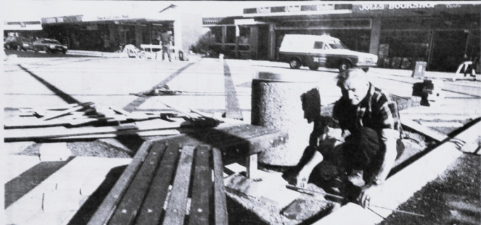
CONTRACTOR for the new shopping precinct in Taradale's Gloucester Street Mr Keith Hulena helping install seats as the work reached its final stages this week.
