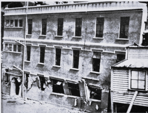
THE earthquake damage to the then newly completed kitchen and dormitory block at Mt St Mary's. The northern end had fallen 1.3 metres. In one of the biggest jacking jobs done in New Zealand to that time, 18 hydraulic jacks, each able to lift at least 50 tons, were brought in to lift the ferro-concrete building and allow the reconstruction of its ground floor.
