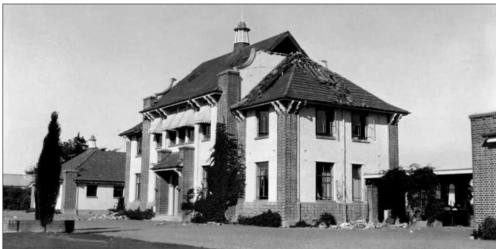
1931 February, Quake damage to roof
