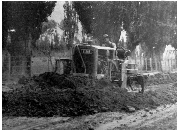
1939 February, A bulldozer making short work of removing spoil from the roadside on Poplar Ave where the highway is being reconstructed
