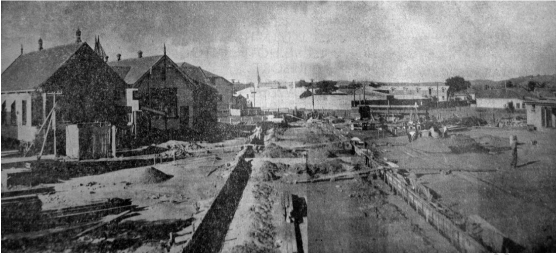
1938 May, Progress on the reconstruction of the new Central School looking towards Warren St shows the old and the new foundations with Drill Hall, council yards and Catholic steeple background
