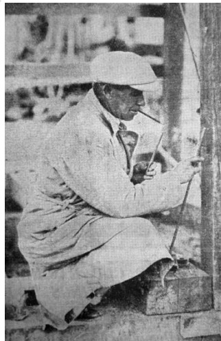
1939, The Clerk of Works tests the first pile driven in for Pakowhai Bridge, an average of 240 blows to drive a pile in but this one took 270
