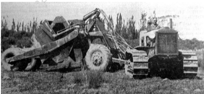
1939 February, Modern machinery, a large bulldozer and scoop now at work on the HB River Boards stopbank scheme at Pakowhai, working at night to complete the stopbanks before winter
