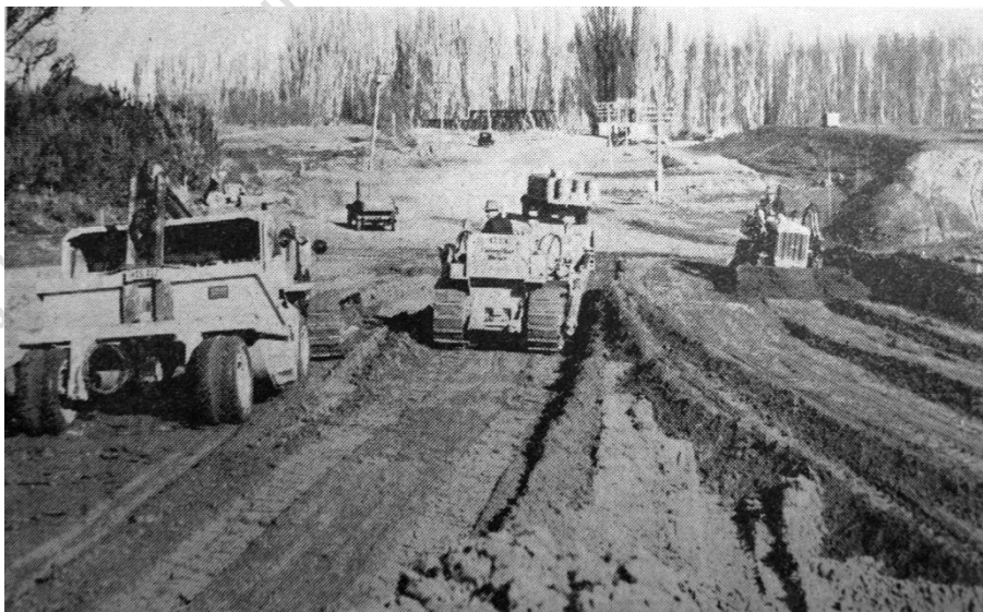
1939, Modern Heavy machinery make light work on the approaches for the new ferro-concrete bridge Pakowhai Bridge, shows the old wooden bridge distant among the trees
