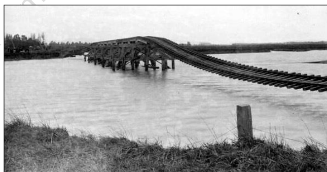
Waitangi rail bridge damaged
