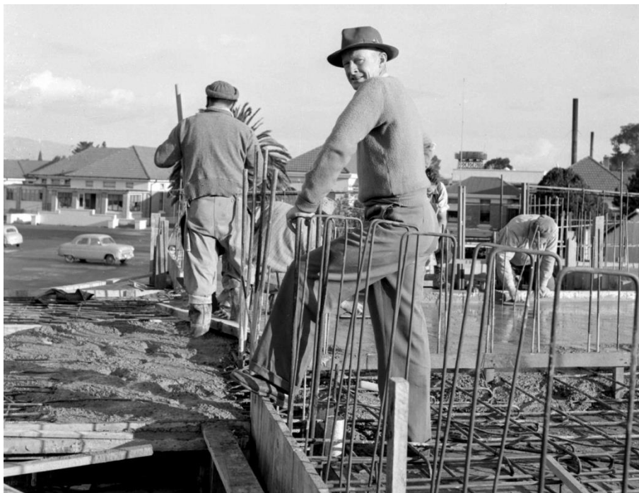
Mr Griffiths, site manager for construction at Hawke's Bay Fallen Soldiers' Memorial Hospital, Omaha Rd Hastings, late 1950s or early 1960s shows tank stand
