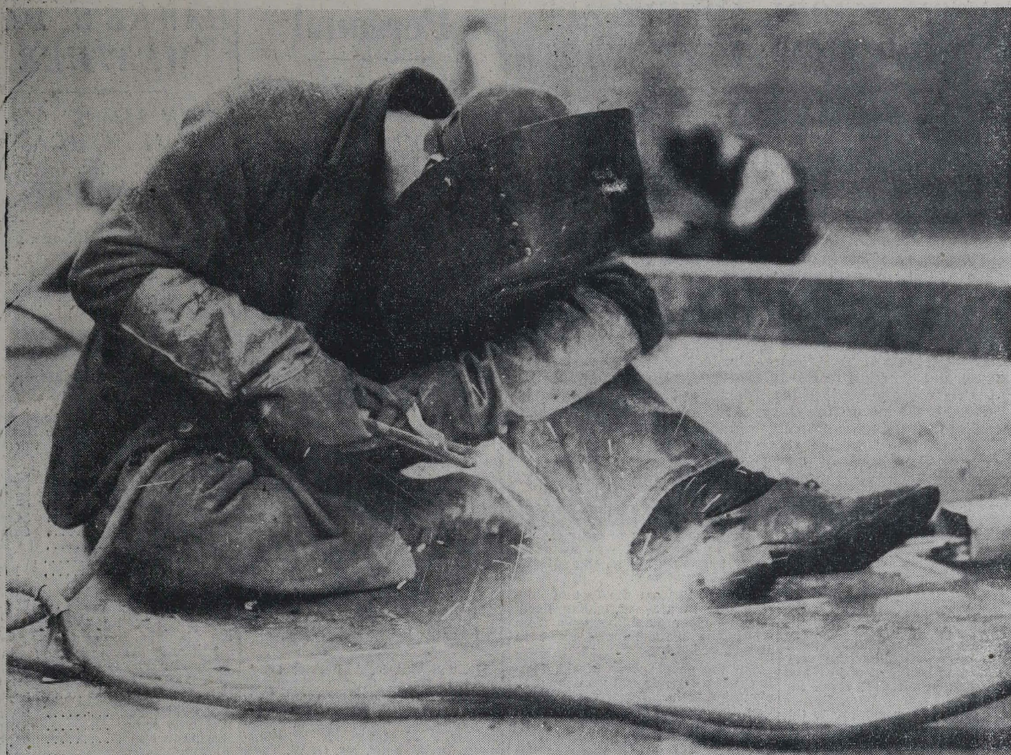
MAN IN THE IRON MASK.—An electric welder bends to his task on the new oil tanks being constructed at Port Ahuriri.
