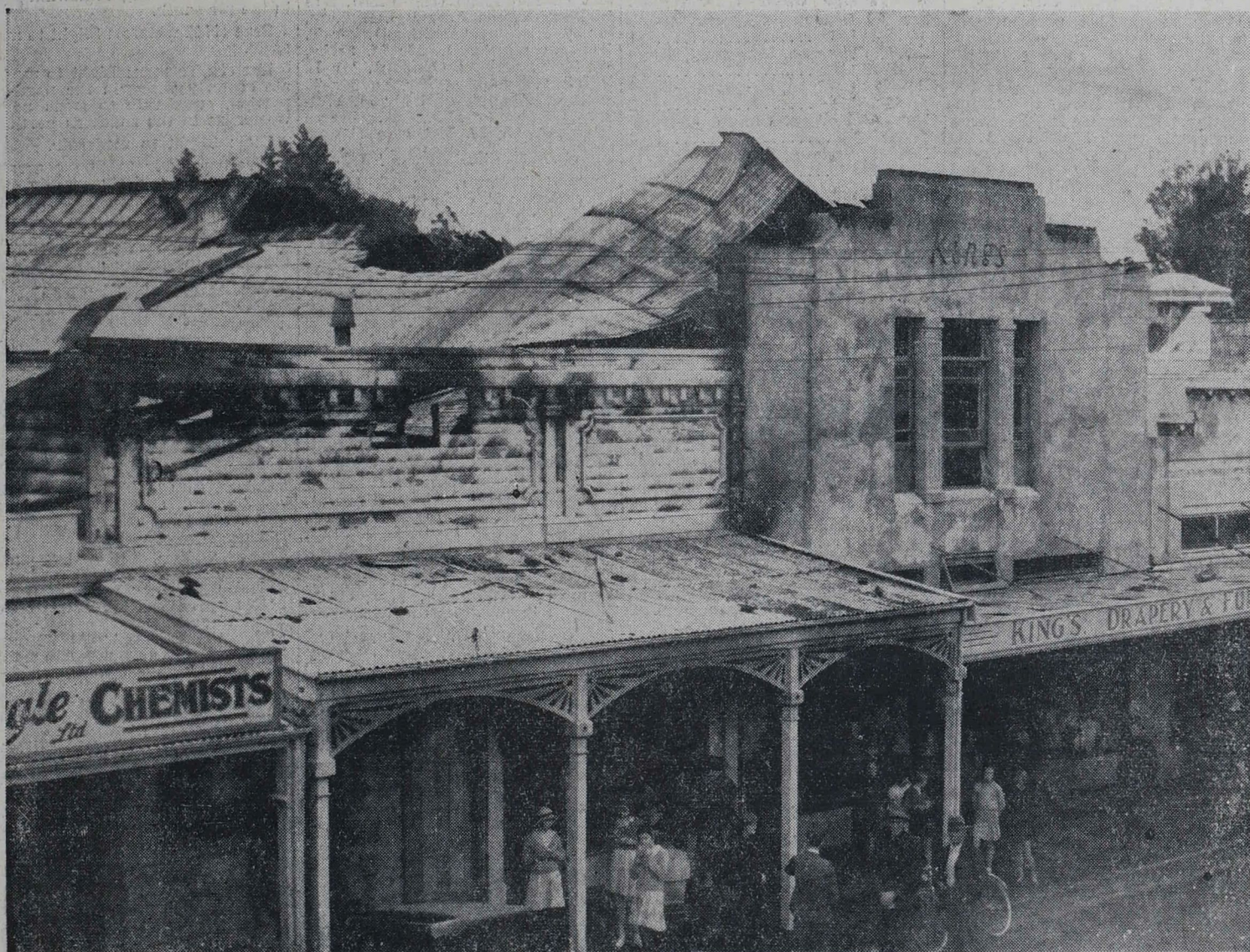
WAIPAWA FIRE BRIGADE.—The sag in the iron roof shows where the flames broke through during the spectacular fire at Waipawa on Friday night, which involved three business premises. Considerable damage was done, the interior of one building and the top floor of another being gutted.
