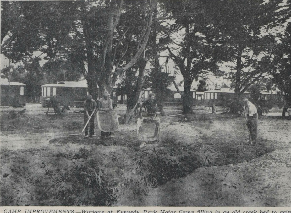
CAMP IMPROVEMENTS.—Workers at Kennedy Park Motor Camp filling in an old creek bed to gain extra space for campers next season. Old tram cabins may be seen in the background.
