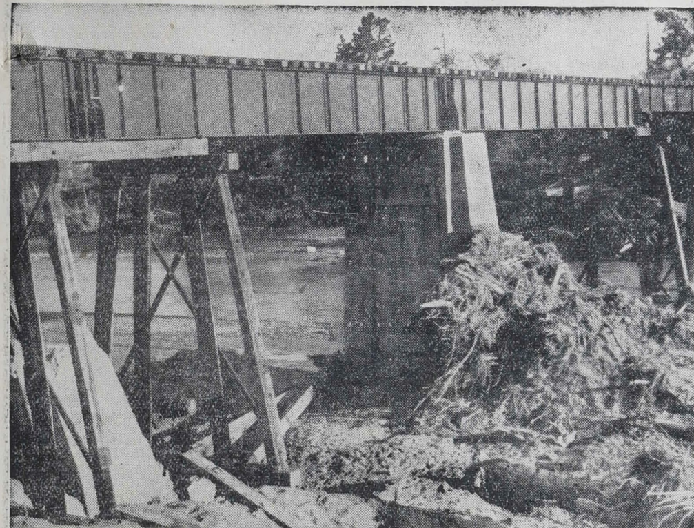
TEMPORARY RAILWAY BRIDGE. —The structure which replaces the bridge destroyed at Wallace's Crossing.
