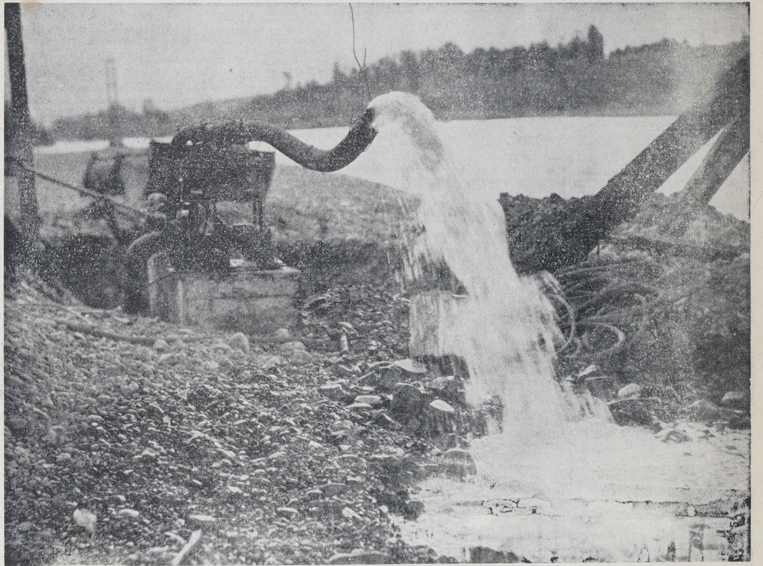
NEW WAIPAWA BRIDGE.—Pumping out water before laying the concrete for the pylons.
