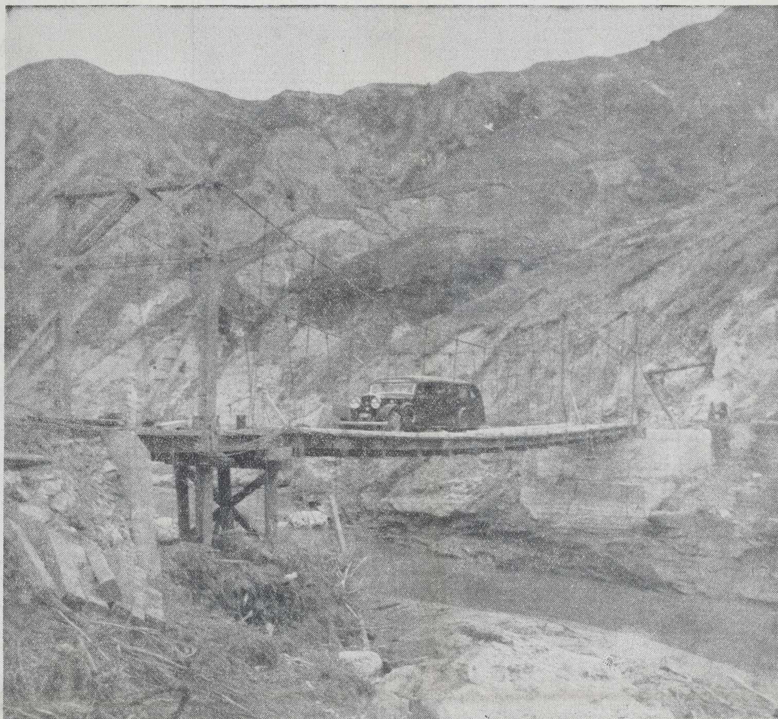
TEMPORARY REPAIRS IN USE RE-OPENING MAIN NAPIER-WAIROA ROAD.—A photograph taken by the "Daily Mail" cameraman this week of the first through service car crossing the temporary suspension bridge over the Waikoau River. This photograph also gives a vivid impression of the slip-scarred country.
