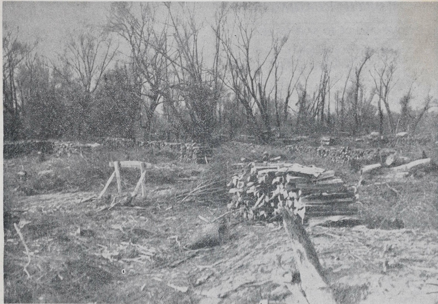
RIVER PROTECTION WORK IS PROCEEDING Apace IN THE HAWKE'S BAY BOARD'S AREA IN AN EFFORT BOTH TO REPAIR DAMAGE DONE BY THE FLOODS AND TO IMPROVE EXISTING PROTECTION WORK.—A series of views taken by the "Daily Mail" cameraman this week during an inspection. The photograph above shows the progress of work in clearing a plantation on the banks of the Ngauroro River. This was so situated that it blocked the last flood and threw the water across country on the other side.
