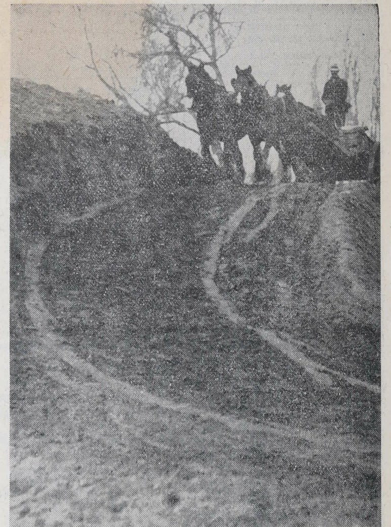
INCREASING THE HEIGHT OF THE STOP-BANK.—A photograph showing work in progress in building the new bank. It will be 17ft. in height—seven feet higher than the former bank.
