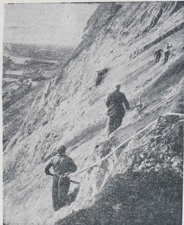
HIGH ABOVE THE WORLD.—Another view of the work proceeding at the Bluff Hill.
