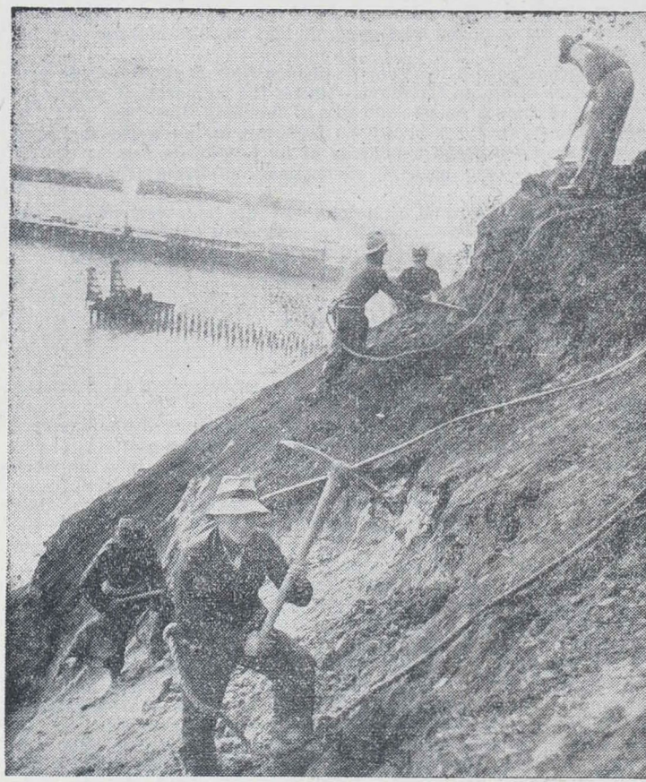
NOT AN EASY JOB.—In spite of the system of safety ropes, few people will envy these men their job on the Bluff Hill. The new pier under construction can be seen in the background.
