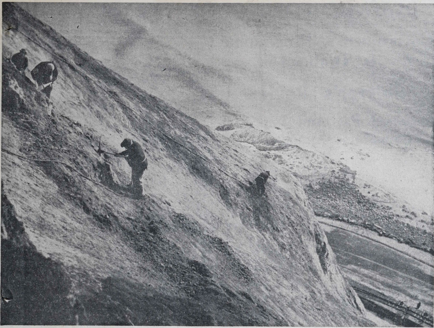
HAZARDOUS WORK.—Regardless of the steep drop to the Breakwater foreshore, workmen are busy trimming the upper face of the Bluff Hill, Napier.
