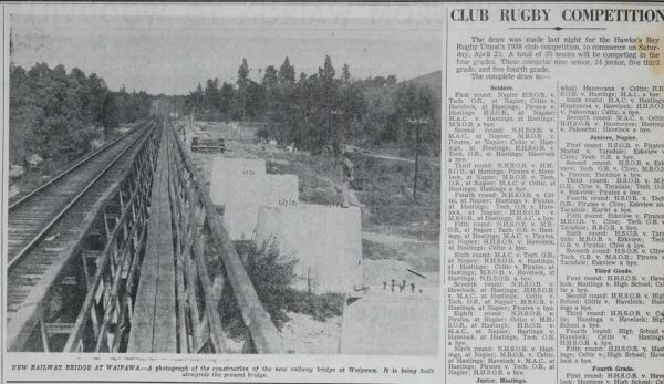
NEW RAILWAY BRIDGE AT WAINOPIA - A photograph of the construction of the new railway bridge at Wainopua. It is being built to complete the present bridge.
