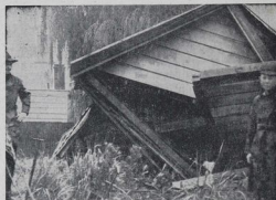
A glimpse of the crushed remains of the house in Mark Street, Napier, which was swept to the down by a huge inundation. Mr. William Lee, the occupant, was severely injured and was taken to hospital.
