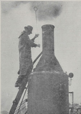
GETTING UP STEAM.—The stoker and with the stoking machinery on the new Pahorahua bridge over the Otaramoana.
