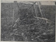
A BLOCKED TRAFFIC BRIDGE.
