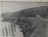
WASHOUTS IN THE ROAD.
