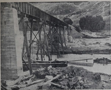
IN THE DEWY OF THE EKE VALLEY.—The fragments of the bridge at Waller's Crossing, which was destroyed in the disastrous floods of April, are now being recovered from the bed of the stream. The present railway bridge, which was hurriedly erected to replace the large bridge, can be seen in the picture.
