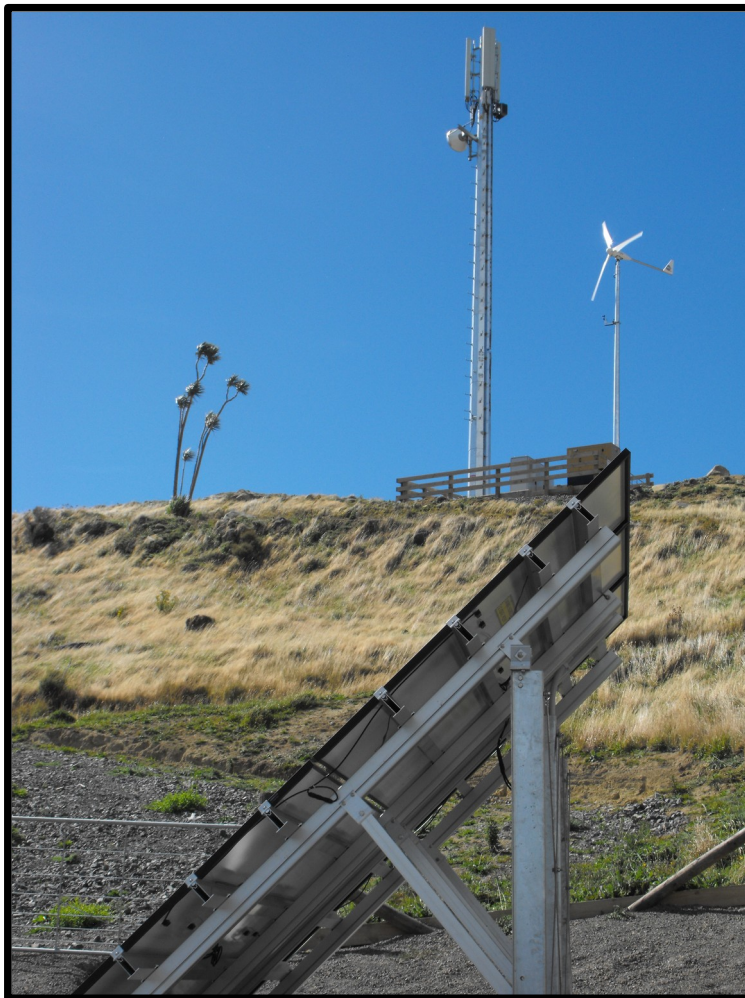
Solar, Wind and Diesel Generator powered cellphone site, East of Dannevirke
