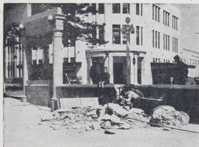
THE COLONNADE.—Work in progress on the Marine Parade Colonnade extension at Napier.
