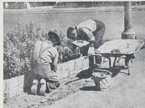
BEAUTIFYING HASTINGS—Workmen building a decorative stone wall round the gardens at Cleo Gibson.
