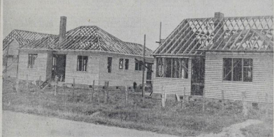
BUILDING OF STATE HOUSES CONTINUES—This group of houses is being built under the State housing scheme in Danversville.
