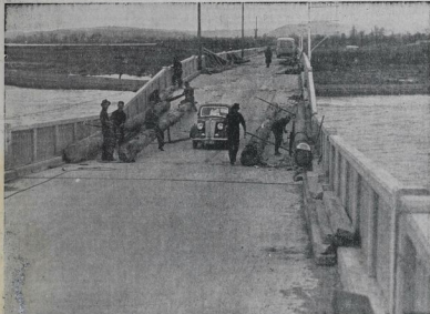
MASS TRAFFIC BRIDGE REPAIRS ADVANCING.—From to-day on traffic will be allowed over the damaged Waikato bridge on the main road to Wairoa, Otago and Whangarei. These heavy beams are to be used as a base on which the pier-drops will work.
