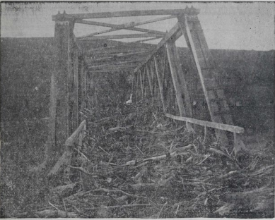
THE ONLY REMAINING SPAN OF THE MOHAKA TRAFFIC BRIDGE, DESTROYED BY THE FLOOD.—This photograph vividly shows the terrific quantity and weight of debris brought down by the flood.
