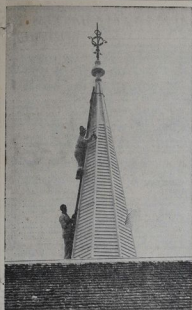
GETTING UP IN THE WORLD.—Painters at work on the steeple of the Anglican Church, Napier.
