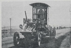
RESURFACING THE MAIN NAPIER-HASTINGS ROAD.—Four miles of the work is progress at this date, where the A. & S. is busy to keep posted by a new process. The tough new heavy surface is being laid in one mile and a half, from the bridge to the commencement of the concrete on the 2 1/2 mile gap.
