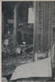
AFTER THE FIRE —An outbreak of fire yesterday afternoon at a house in Progress Street, Hawke's Bay, and considerable damage before it was quelled. This is the back portion of the building, where the fire originated.
