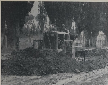
RECONSTRUCTING A ROADWAY —A bulldozer makes short work of removing spoil from the roadside in Poplar Avenue, where the highway is being reconstructed.
