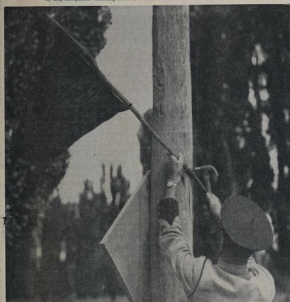
WARNING TO MOTORISTS —An Automobile Association officer putting up a temporary warning to motorists while the road through Poplar Avenue, Ashburton, is being reconstructed.
