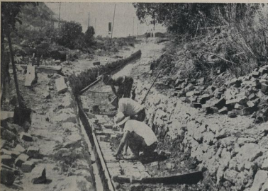
DRAGS OUT OF RANTZQVIST DESIRE.—The Napier Borough Council is constructing a rock garden watercourse at a point near the Rantzqvist development.
