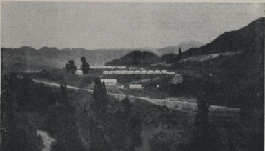
THE BEAT OF A NEW POWER SCHEME —The Number 2 Construction Camp at Puke, where the majority of the 200 men engaged on the new scheme. Work completed (clockwise from top) the East Coast Scheme will suggest the supply of electricity from Westland to the Bay of Plenty. An original line covering the area of the scheme is shown above the area, and a 2500 ft cable air raised between the works in progress.
