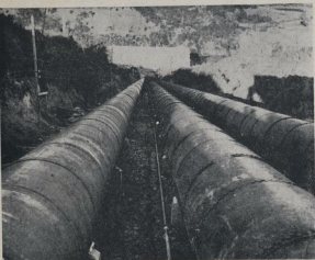
WAIKAREMOANA'S PIPELINES. —These great pipes, eight feet in diameter, carry the water from the lake to the power station at Teai, for delivery.
