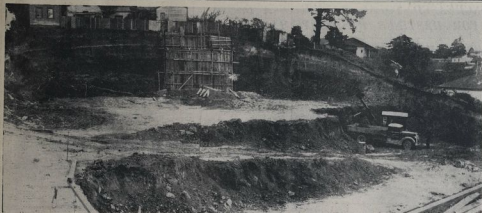
A BIG DITCH —Work is proceeding steadily with the construction of the new reservoir at Napier. The scaffolding and planting in the background have been erected as a starting point for erecting concrete.
